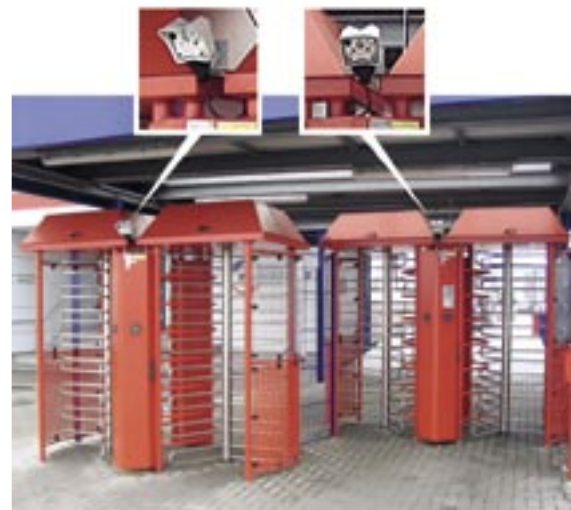
Network surveillance cameras at entrance areas
